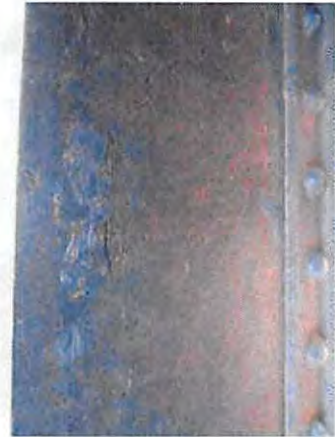
75-NCRRR Ped Bridge_Y14_L7L8 South interior plate flaw
