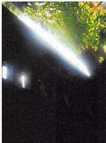
107-NCRR Ped Bridge_Y14_Timber split
