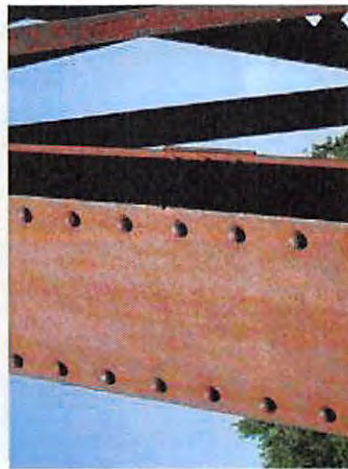
80-NCRRR Ped Bridge_Y14_U1L0_North scrapes
