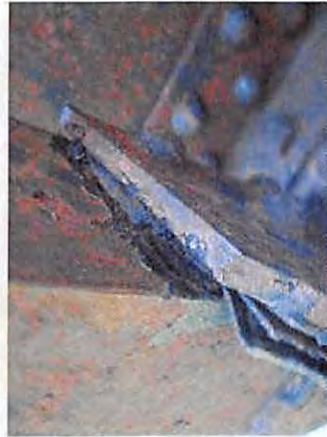
74-NCRRR Ped Bridge_Y14_L7_South east pack rust loss
