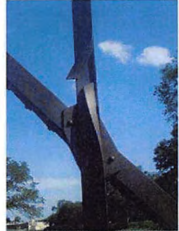
120-NCRR Ped Bridge_Y14_U1L1 South tear
