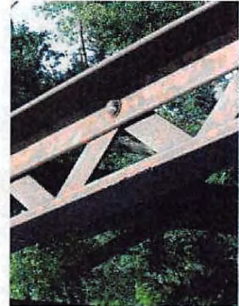
66-NCRR Ped Bridge_Y14_U3L1 South interior scrapes
