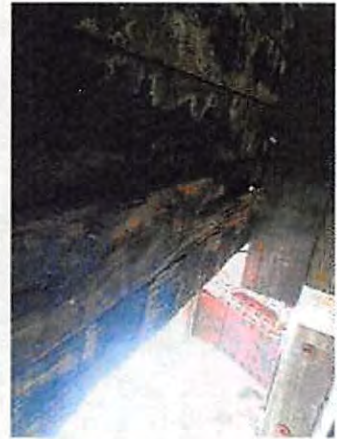
105-NCRR Ped Bridge_Y14_Timber jump span deterioration
