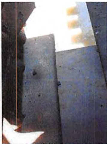
43-NCRR Ped Bridge_Y14_Typ. lower chord pitting at connections
