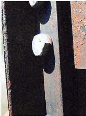
68-NCRR Ped Bridge_Y14_U3L5 South crack
