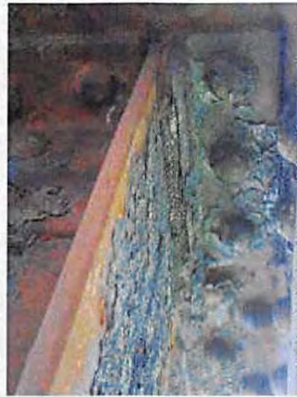
101-NCRR Ped Bridge_Y14_Typ. Pack rust under stringers
