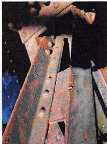
53-NCRR Ped Bridge_Y14_U5L7 North scrapes
