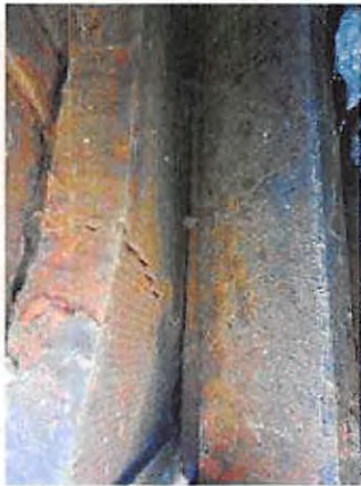
94-NCRRR Ped Bridge_Y14_L0 South bottom plate crack
