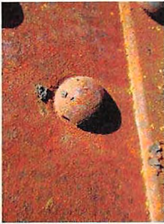
10-NCRR Ped Bridge_Y14_U4 North Rivet, typ. impact
