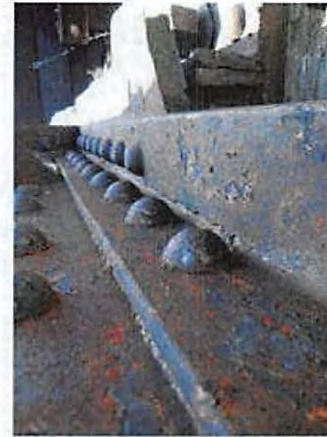
93-NCRRR Ped Bridge_Y14_L0 North Exterior angle crack
