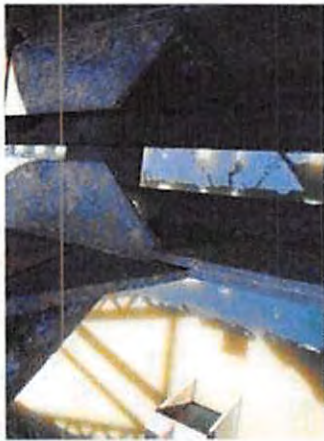
40-NCRR Ped Bridge_Y14_L2 North west exterior diagonal pack rust
