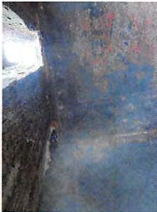
46-NCRR Ped Bridge_Y14_Typ. stringer connection rust
