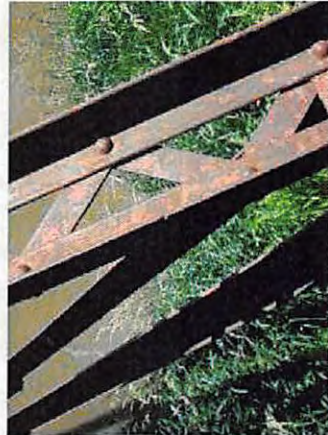
65-NCRR Ped Bridge_Y14_U3L1 South interior scrapes
