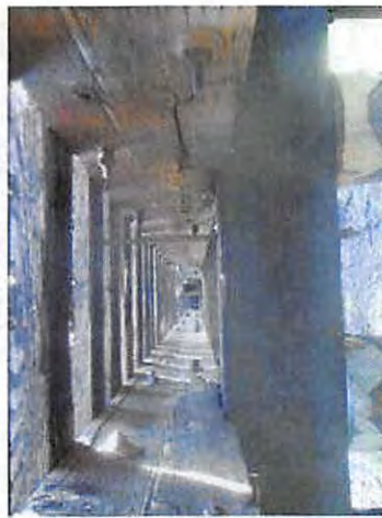
113-NCRR Ped Bridge_Y14_Timber deterioration
