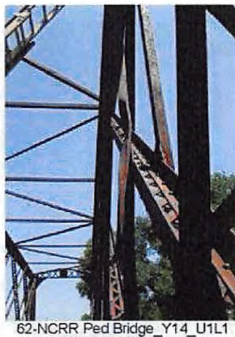
62-NCRR Ped Bridge_Y14_U1L1 South interior torn at diagonal connection
