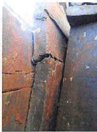
92-NCRRR Ped Bridge_Y14_L0 North bottom plate crack
