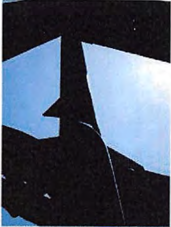
64-NCRR Ped Bridge_Y14_U1L1 South interior torn at diagonal connection
