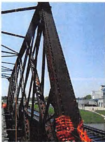
61-NCRR Ped Bridge_Y14_U7L8 North Missing Rivets and new bolts
