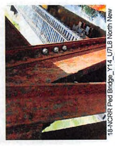
18-NCRR Ped Bridge_Y14_U7L8 North New cover plate bolts
