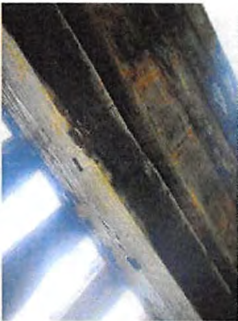
106-NCRR Ped Bridge_Y14_Timber corner loss
